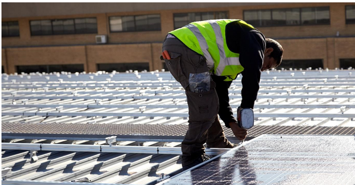
Installation of rooftop PV (© GreenCape. Images reproduced with permission from GreenCape)
