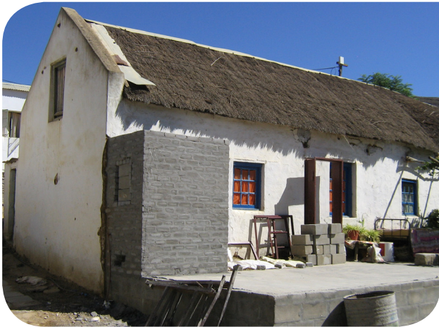
FIG.1.51 EXTERNAL BLOCK TOILETS IN WUPPERTAL - SPOILING HISTORICAL FRONTAGES
