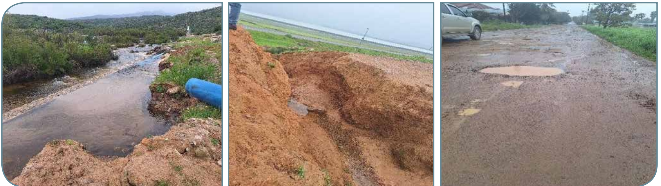
Figure 50: Cederberg Municipality damages
