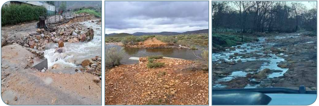
Figure 54: Breede Valley Municipality damages
