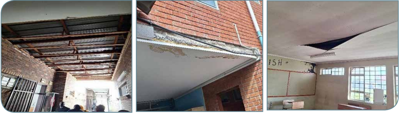
Figure 60: Department of Education damages
