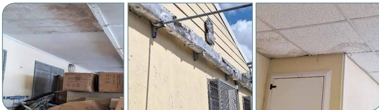
Figure 59: Department of Health and Wellness damages
