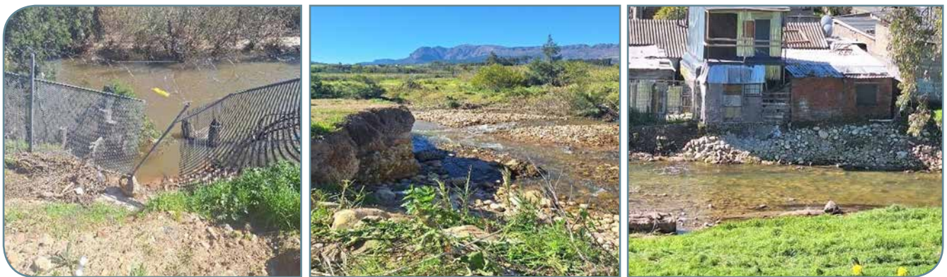
Figure 57: Drakenstein Municipality damages
